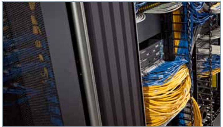
Figure 8. Effective cable management in high-density configurations must prevent stress on cables and connectors.
